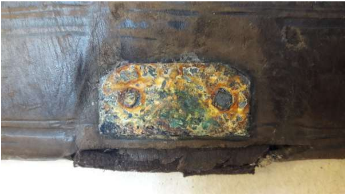
Photo 26 PDC222. Detail of the metal plate that held the leather strap. Part of the leather strap is stil visible along with the corrosion of the metal.
