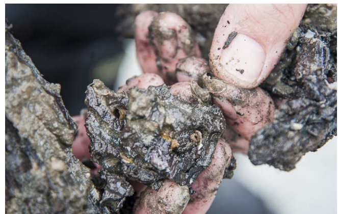
Fig. 3.34 Wood from the BZN 18 site completely eaten and crumbled due to Teredo attack. Photo: Paul Voorthuis, Highzone Fotografie.
